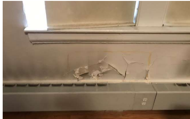
Deteriorated Interior Finishes (Water Leakage)
