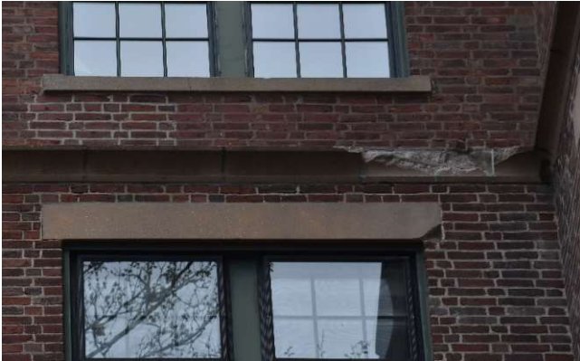
Spalled Cast Stone
