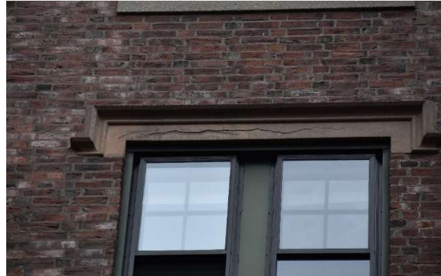
Cracked/Spalled Cast Stone
